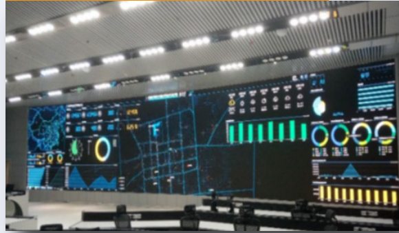
Control & Command Centre
